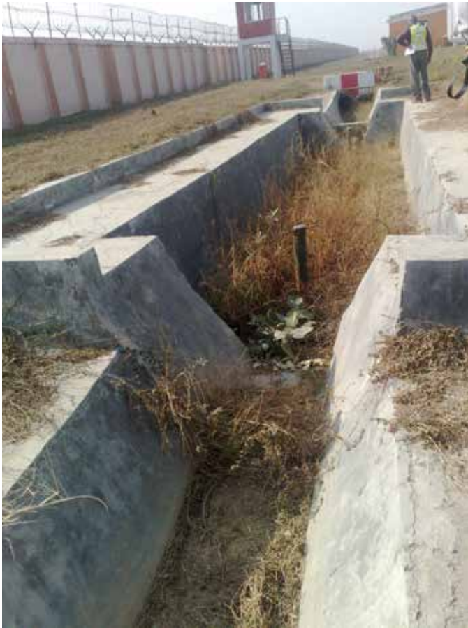
Figure 7. A groundwater recharge structure in the storm water drain, International Airport, Delhi.
