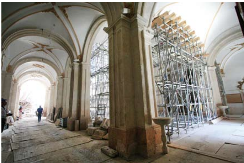
Figura 29. Apeo de los arcos formeros de la nave central de la Iglesia de Santiago. Figure 29. Propping up of the arches over the nave of the church of Santiago.
