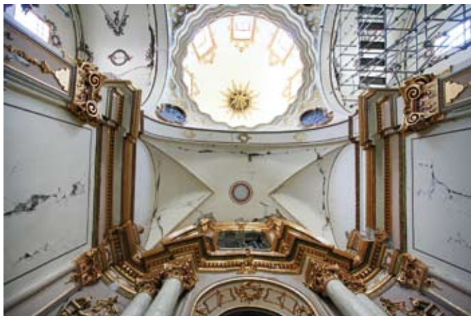
Figura 27. Apeo de los arcos del crucero de la Iglesia del Carmen. Figure 27. Cracks in vaults and the cupola of the church of the Carmen.
