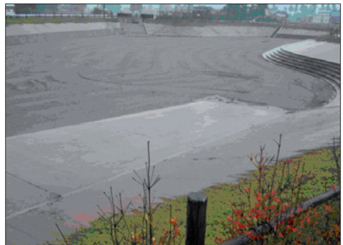
Figure 2. Toyama Prefecture's infiltration basin No.2, Oct. 08, 20093. The Rokugo alluvial fan, Akita Prefecture
