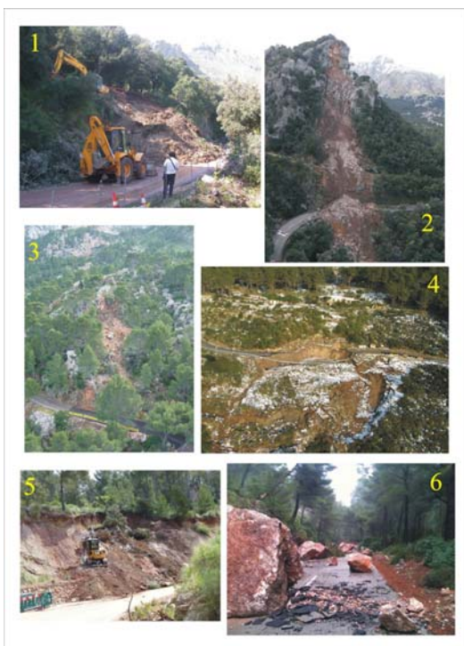
Figure 1 Photographs of the most important movements affecting the Ma-10 road. 1) Sa Calobra (3/12/2008), 2) Gorg Blau (31/12/2008), 3) Estellencs (15/01/2010), 4) Estellencs (8/03/2010), 5) Banyalbufar (09/05/2010) and 6) Pilar (12/10/2010).
