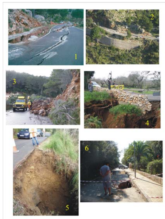
Figure 2 Photographs of secondary roads on the range affected by landslides and karstic collapses (sinkholes). 1 and 2) Cala Tuent landslide (15/12/2008), 3) Es Verger landslide (15/12/2008), 4) Búger sinkhole (Jan 2010), 5) Es Verger sinkhole (15/12/2008) and 6) Crestatx sinkhole (3/5/2010).
