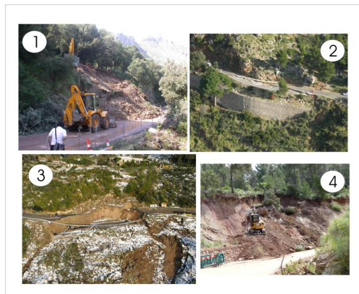
Figure 2 Photographs of the most important landslides recorded that affected the road network in the mountain range. 1) Sa Calobra (3/12/2008), 2) Cala Tuent (15/12/2008), 3) Estellencs (8/3/2010) and 4) Banyalbufar (9/5/2010). The Estellencs landslide cut off the Ma-10 road for 3 months.
